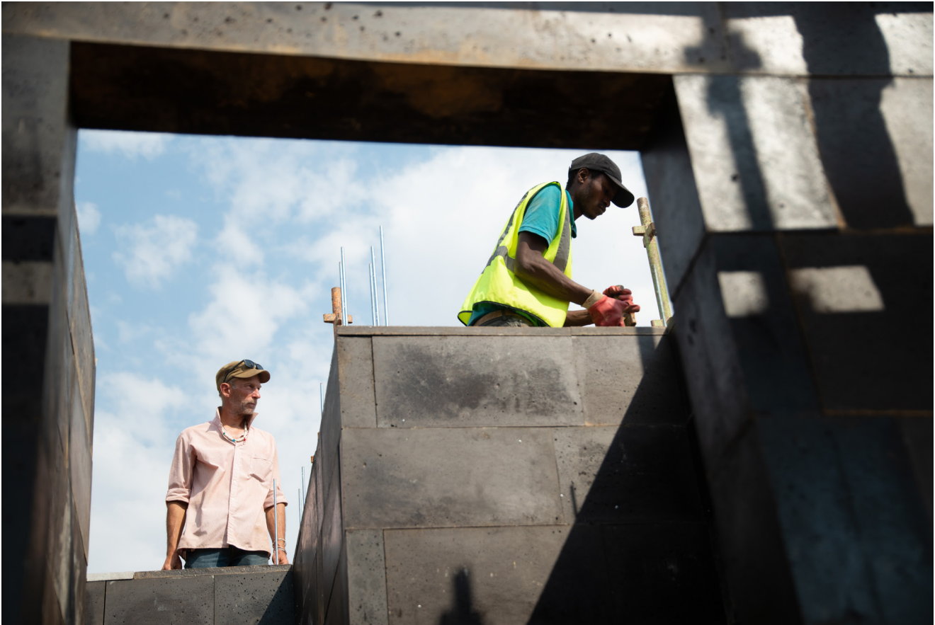
The SBIR project is on site in Namibia: building with polyblocks made from foundry sands.
